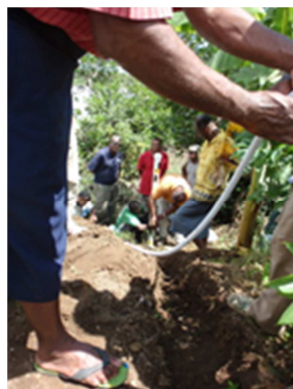
Cable in casing tube (Fiji 2011)
