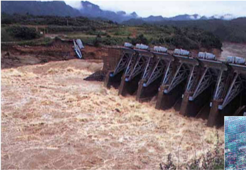
Collapse of Yeoncheon Dam
