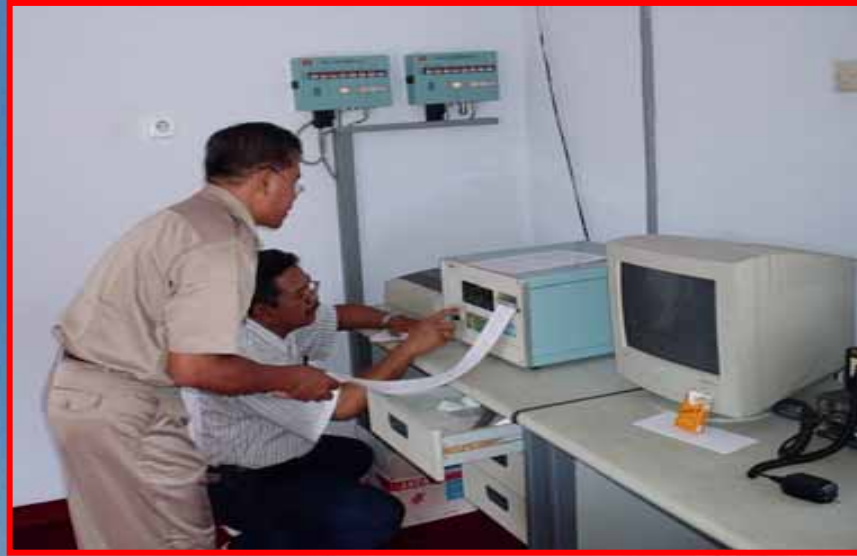
Main Control Station of Lahars Warning System in Lumajang
