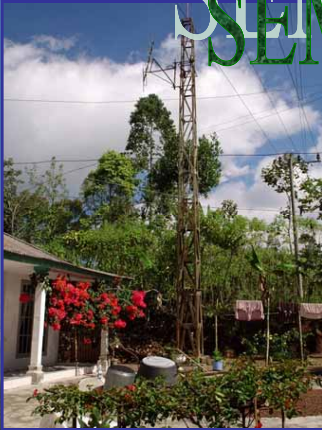
Station of Lahars Warning System in Lumajang
