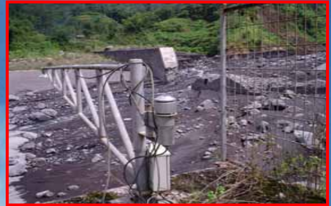
Telemeter System of Automatic Water Level Recorder in Besuk Koboan River
