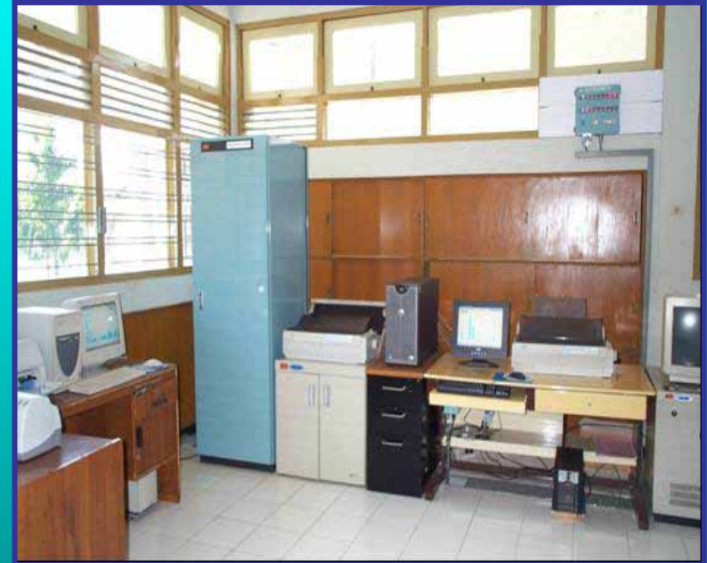
Control Room of Telemeter System in Experimental Station for Sabo in Yogyakarta
