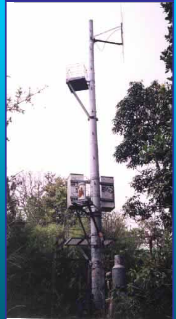
Telemeter System of Automatic Rain Gauge in Plawangan
