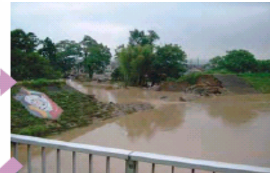
Broken point of the embankment
